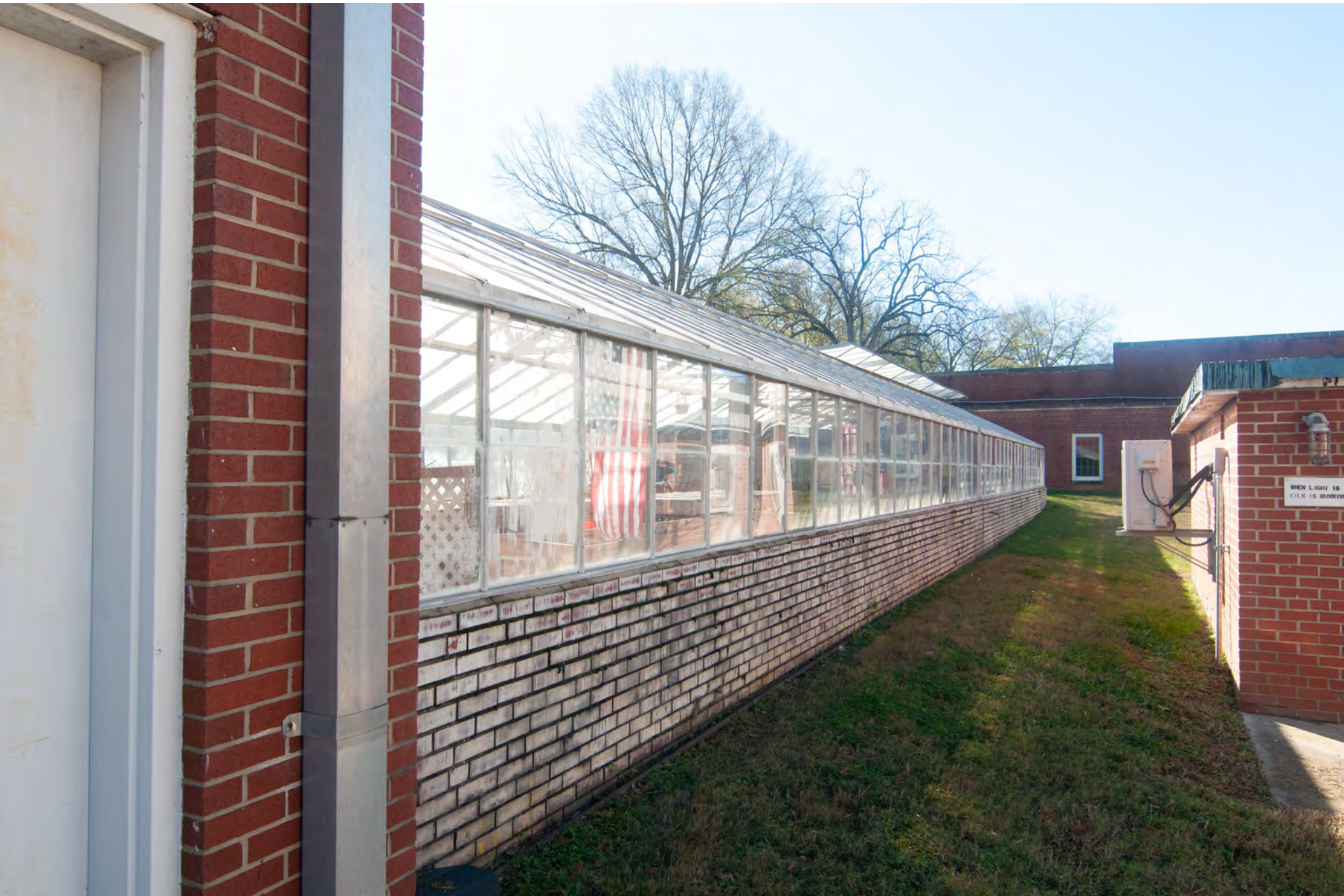
Photo 42 of 55.Salisbury VA Hospital Historic District, Salisbury, Rowan County, North Carolina. March 2021.
