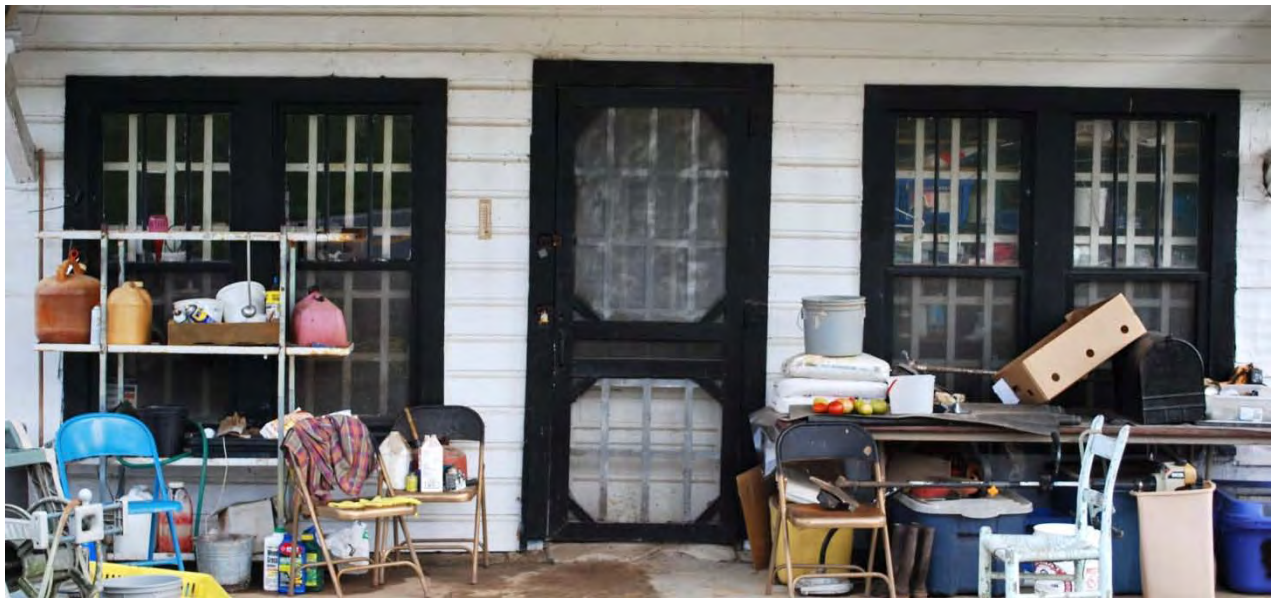
BK0365, Grover S. and Viola Holland Store, 1942, 1960, 5285 US 64, Morganton vicinity Metal security bars inside front door and windows
