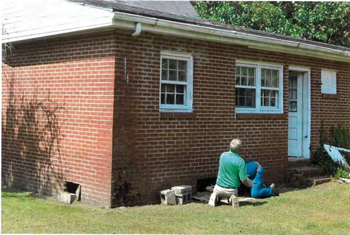
Fig. 22. Northeast corner – water staining from missing downspout and biological growth on wall.
